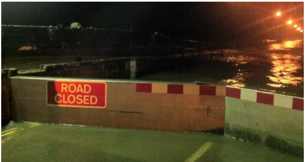
Image 2: Highway flood gate located in Instow, North Devon – Picture ITV Westcountry
