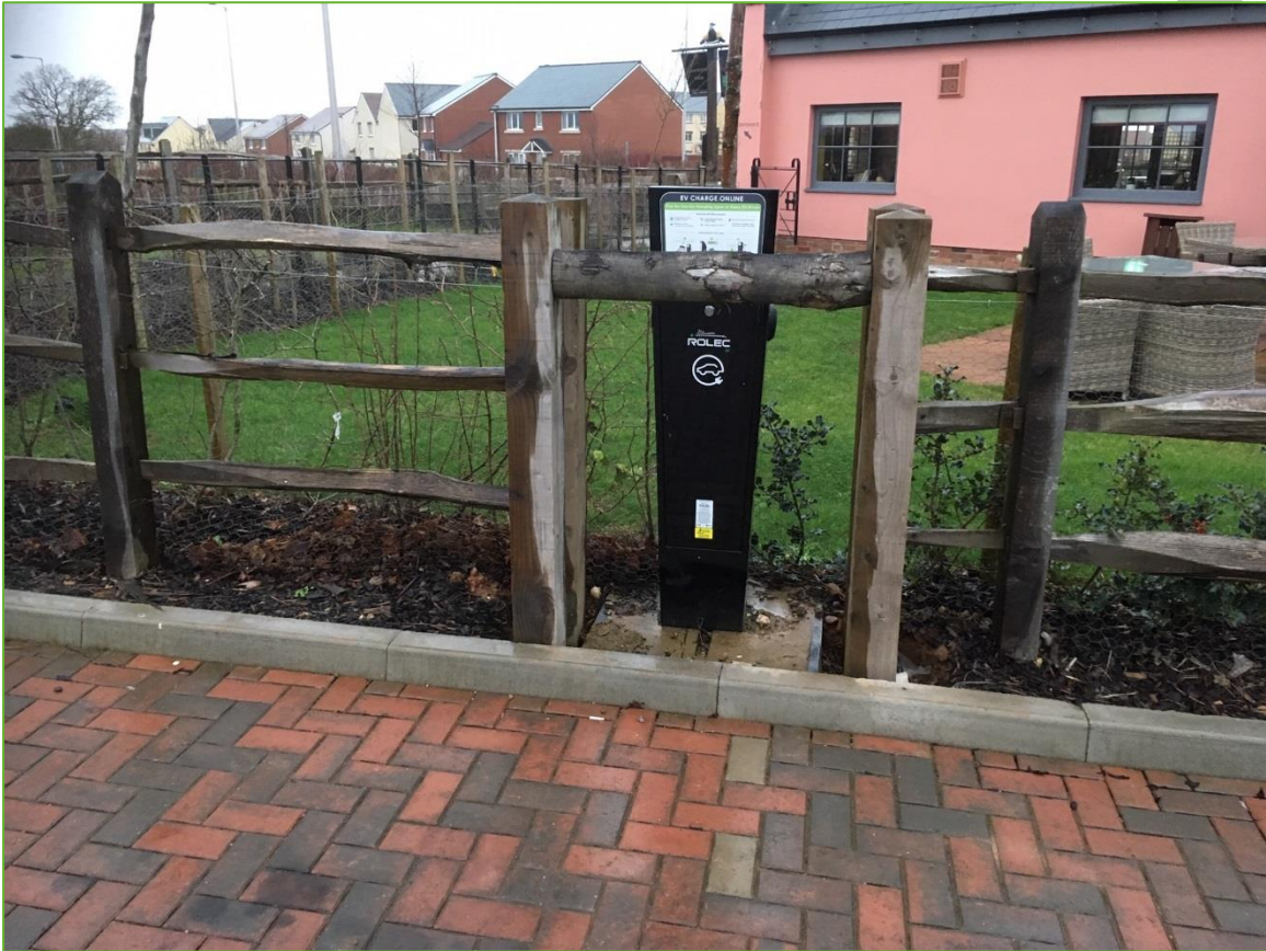
Figure 10 – existing EV charging at Cranberry Farm, Cranbrook
