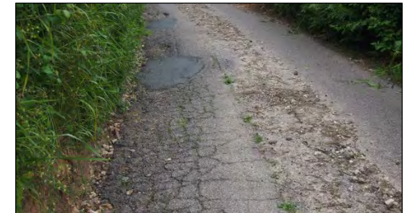
Damaged road surface, Otter Valley
