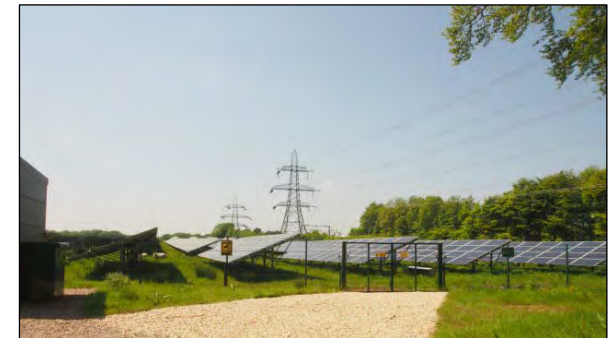
Solar Farm east of Axminster.
