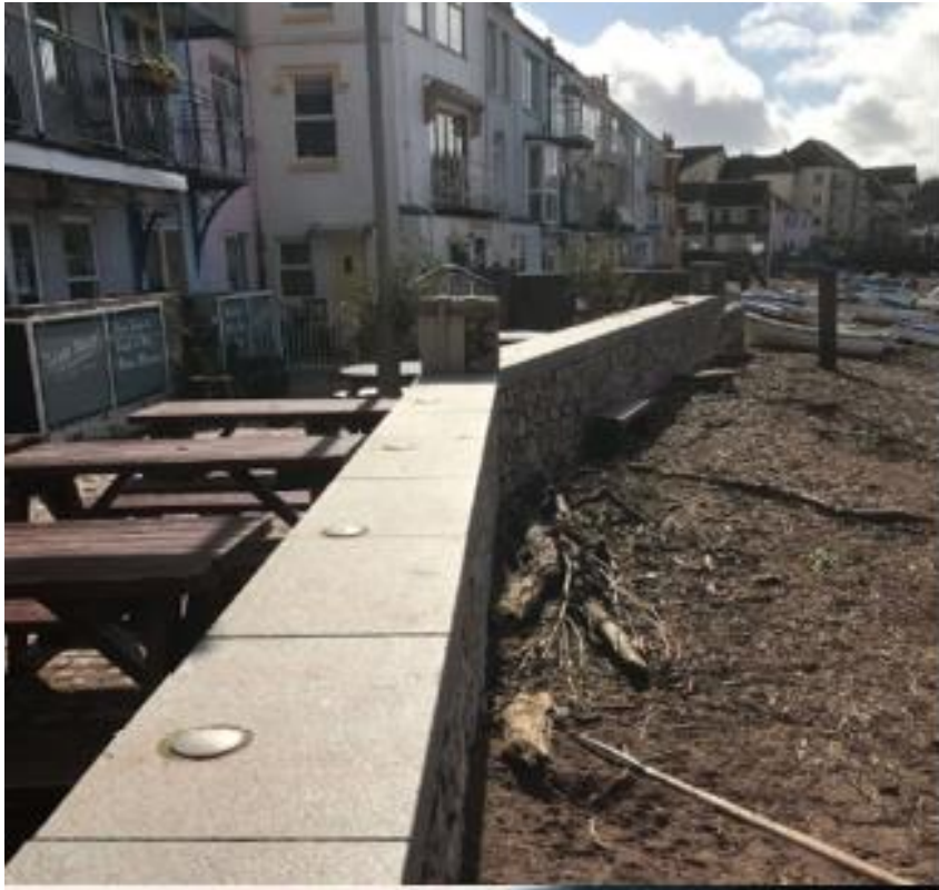
Above: Teignmouth Back Beach Wall under normal conditions. Note stone clad front, and rendered rear. The change in direction requires a permanent post.
