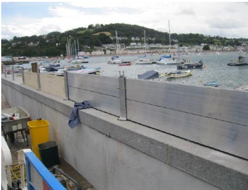
Above: Teignmouth Back Beach wall under storm event conditions. Note photo taken during initial installation, as top up sections not yet used under storm conditions.
