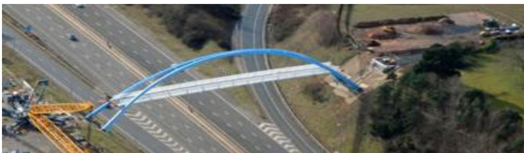
Redhays bridge spans the M5 providing a link for cyclists and pedestrians
