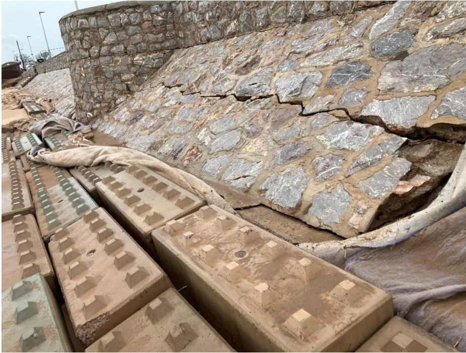
Image 1.5. Wall damage and temporary repairs.
