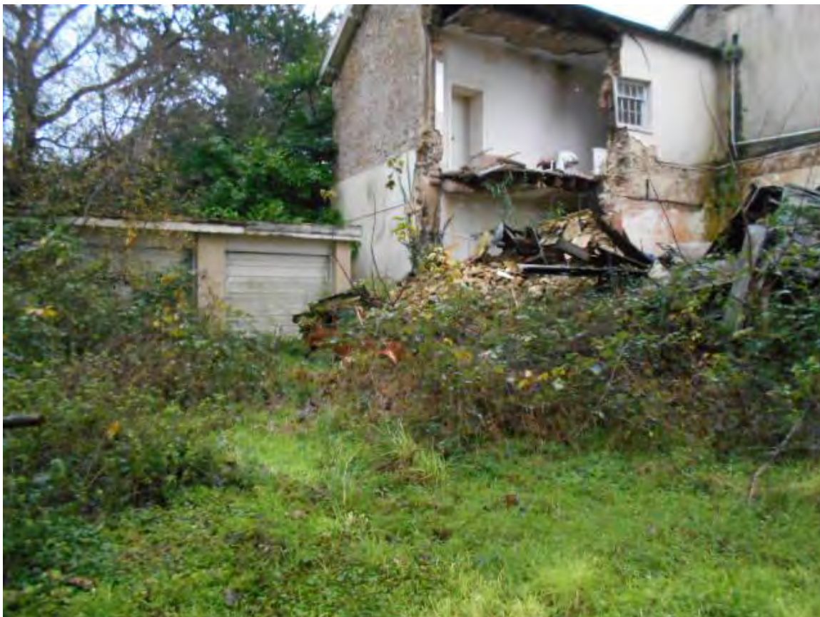
The Wing – showing the most recent deterioration and collapse.
